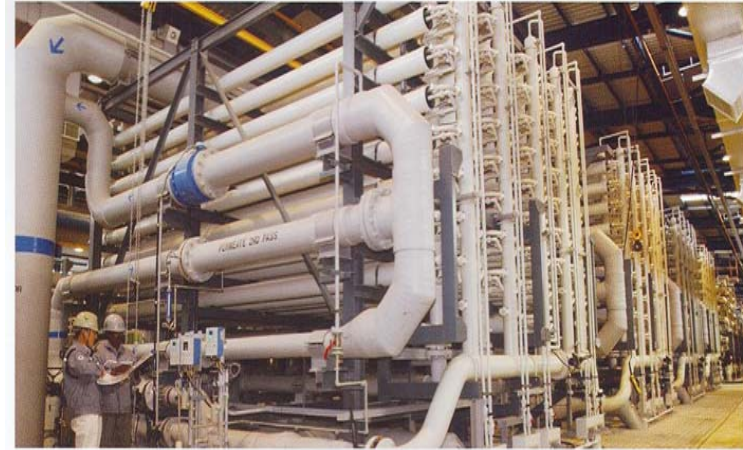
Fuairah Water & Power Plant
